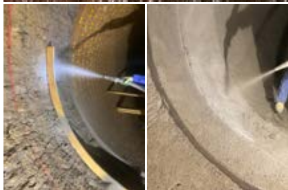
North Rhine-Westphalia: (top) old brickwork, almost dust-free gunning with field classification. (Bottom) final result after installation.
