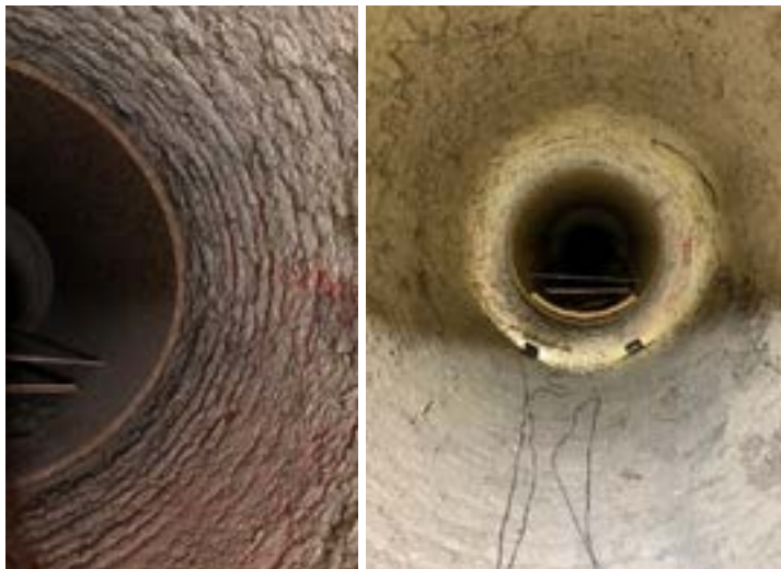
Premature wear of MgO/Spinel bricks.
